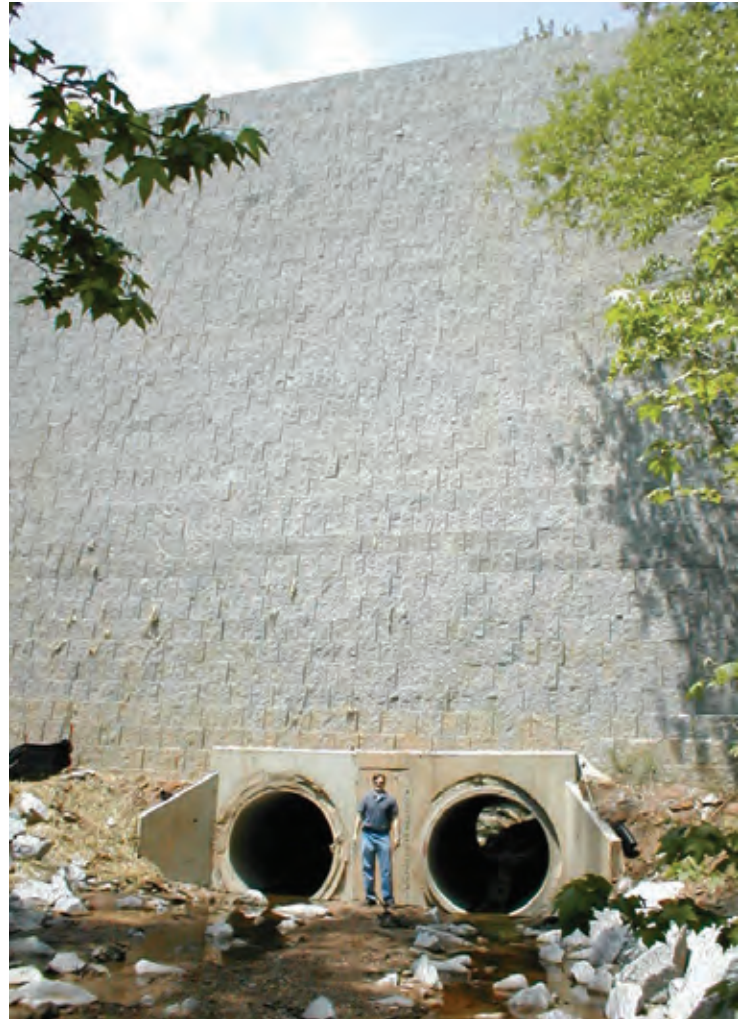
To provide drainage, this land bridge structure has two 6-foot-diameter culverts through the 61-foot-high walls.
