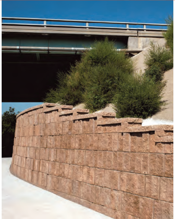
The Landmark® retaining wall system was the cost-effective solution to completing this 5-mile-long trail project. Nearly 30 percent of the project was installed with direct anchorage, which made it possible to complete the project without closing adjacent roadways.
